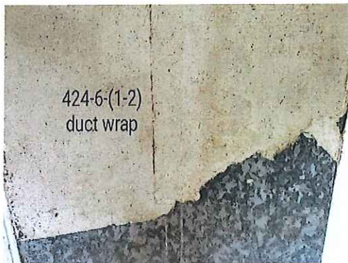
424-6 Duct wrap Typical interior 30% Chrysotile
